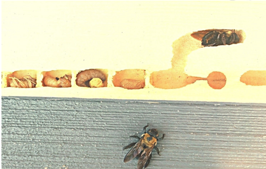
Carpenter bee gallery and damage to fascia board
